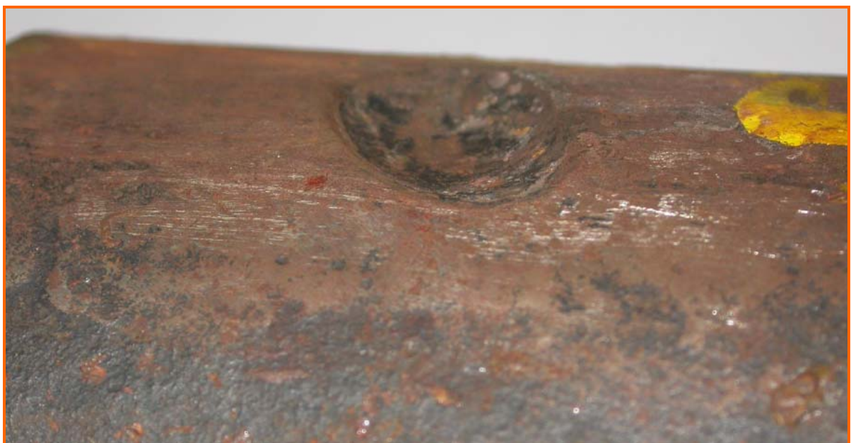
Fig.3: Close-up view of area with local wall thinning.
